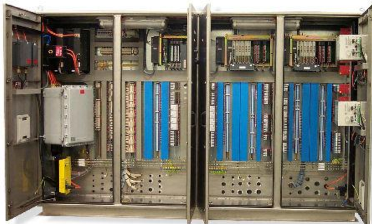
Compressor control system for F.P.S.O. executed in Exp (Ex p de (ia)(ib) IIB T3
